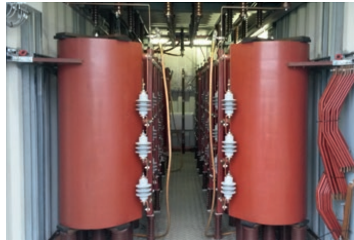
Insight of a measurement container for a certification campaign in the field
