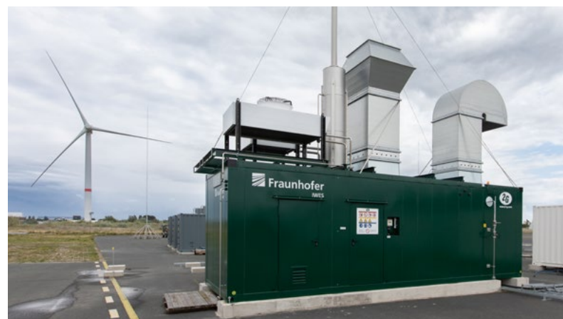
Hydrogen CHP at the HLB testing area with the AD8-180 offshore wind turbine prototype in the background.
